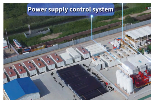
WELL-SITE POWER SUPPLY
